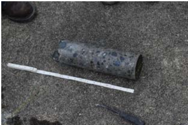
Fig. 11 : Concrete core from “Green area”
