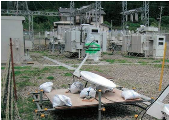
[Transportable VSAT Station deployed at Ootsuchi Substation]
