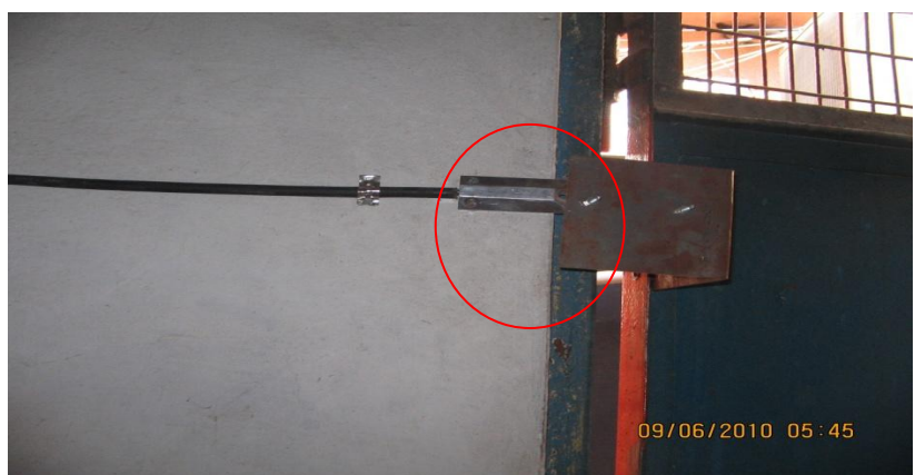
DOOR SENSOR at SITE
