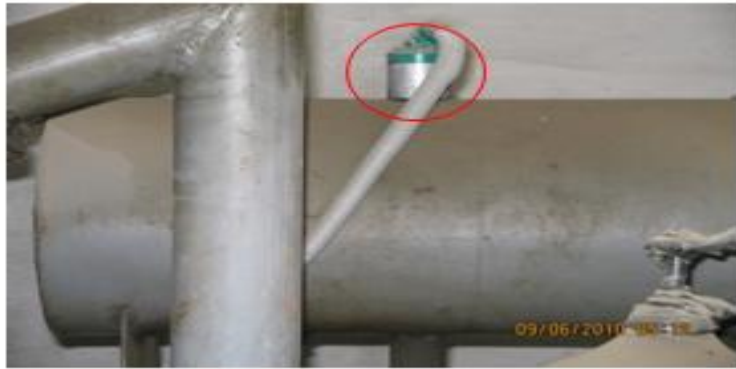
OIL LEVEL SENSOR at SITE
