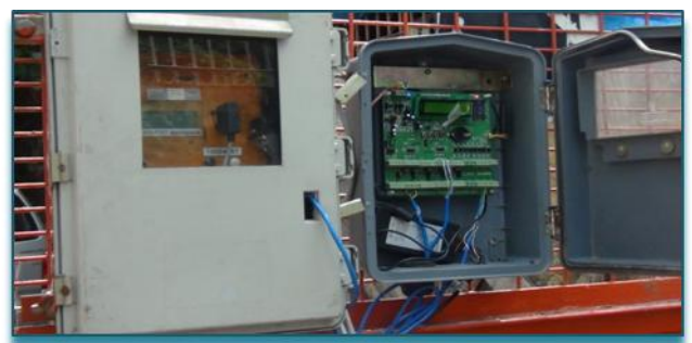
METER AT SITE
