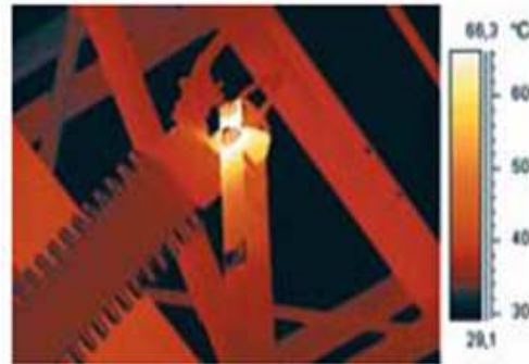
Incorrectly secured connection
