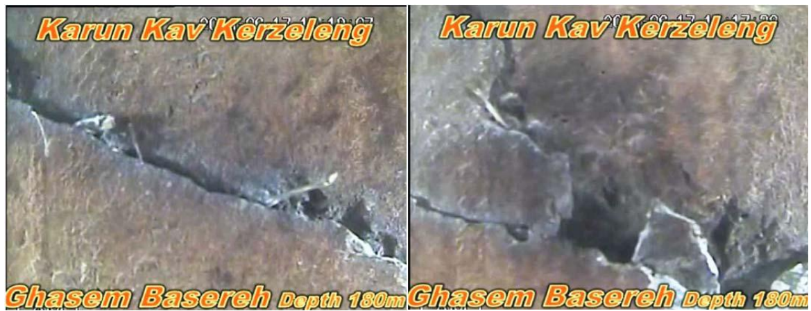
Figure 11. Crack(s) in blocks 2 and 4 – sample photos from crack outcrop in dam upstream face(2013)
