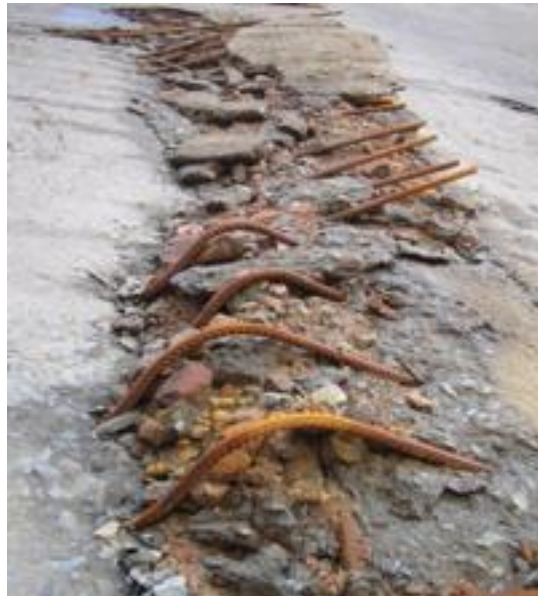
Figure 2 : Pulled reinforcement on the upstream concrete face.
