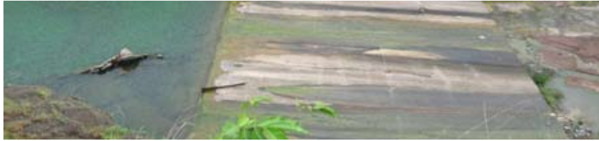
Figure 3. View of dislodged RCC panels in Bhama Askhed dam EDA.
