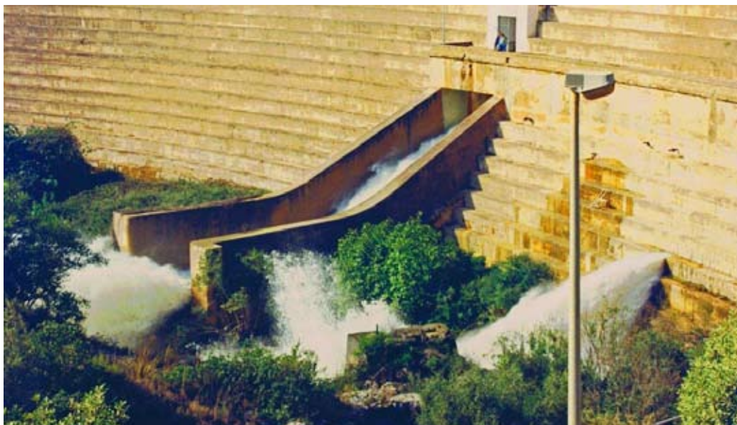
Figure 2 : Uncontrolled outflow next to the bottom outlet detected during overtopping.
