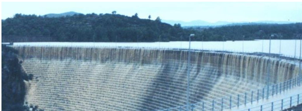
Figure 1 : Overtopping of the dam crest.
