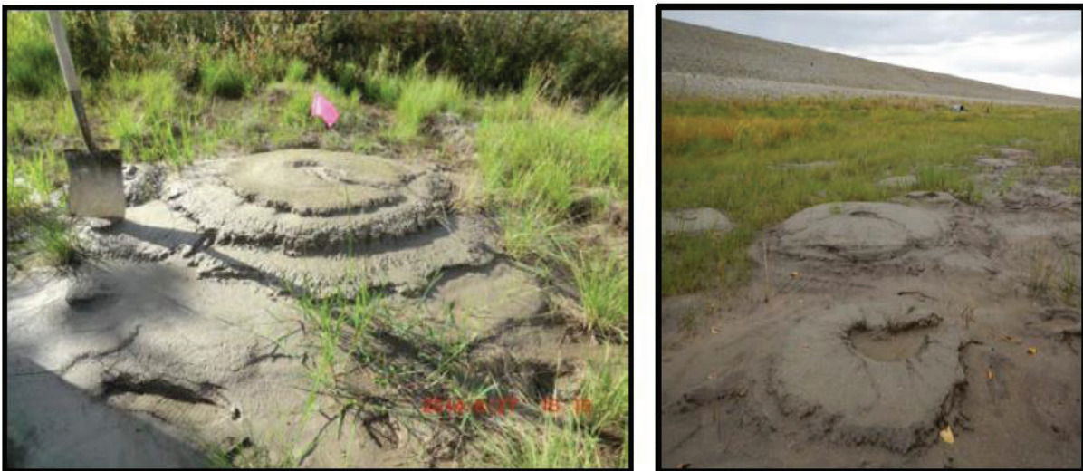
Figure 3 : Sand boils observed downstream of Moose Creek during 2018 floods.
