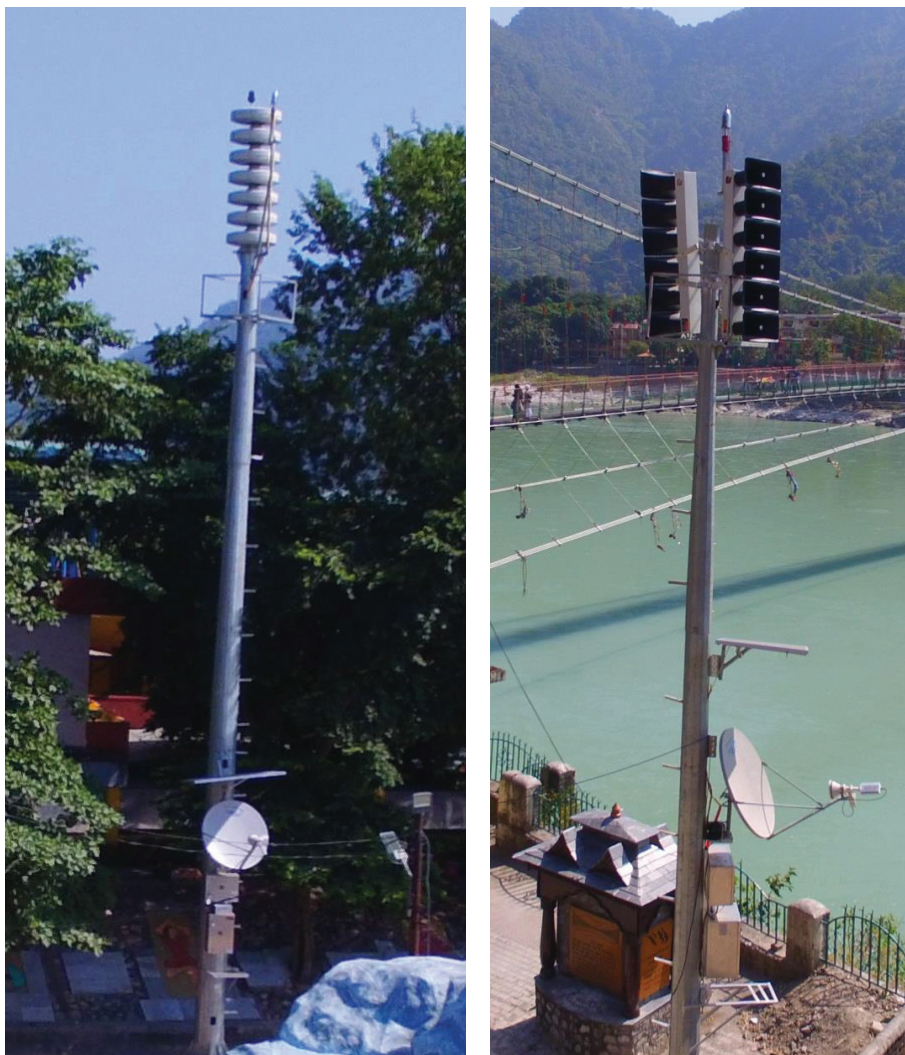
Installation of Legacy Modulator siren in Triveni Ghat and Direction speaker array siren in Ram Jhula
