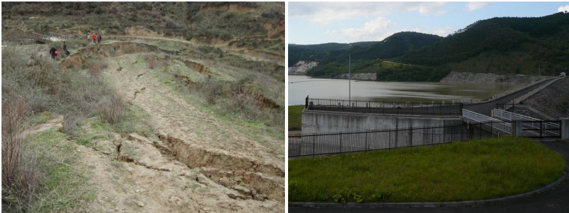
Figure 4. Failure of Sharredushk embankment dam in Albania due to a magnitude 4.1 earthquake in 2009 (left) and undamaged Aratazowa rockfill dam in Japan, which was subjected to peak ground acceleration of 1.0 g during the magnitude 7.2 Iwate Miyagi Earthquake in 2008 (right)
