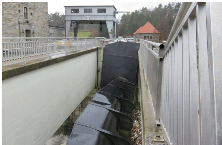
Figure 6 : Inclined and damaged the upper spillway gate in the fourth spillway.
