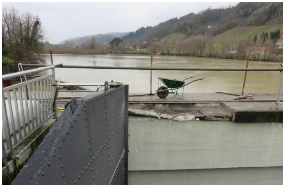
Figure 7 : Damaged concrete beam of the crane rail on the dam's crest (right side of the fourth spillway).
