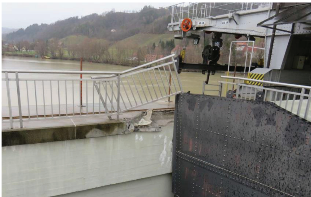
Figure 8 : Damaged concrete beam of the crane rail on the dam's crest (left side of the fourth spillway).
