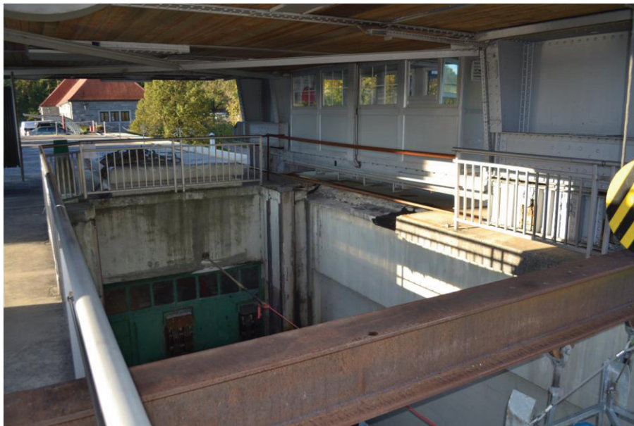
Figure 10 : The start of the second phase of rehabilitation works – disassembly of the upper spillway gate.
