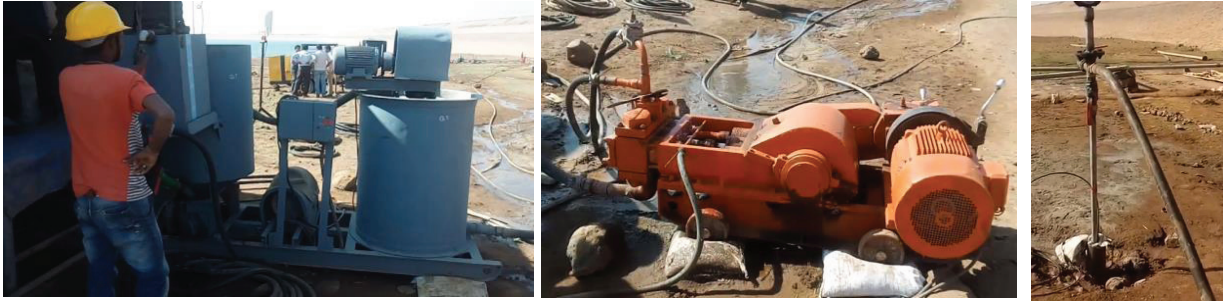
Photo 3 : (a) Mixing of cement with water (b) Developing pressure for grouting (c) grouting location
