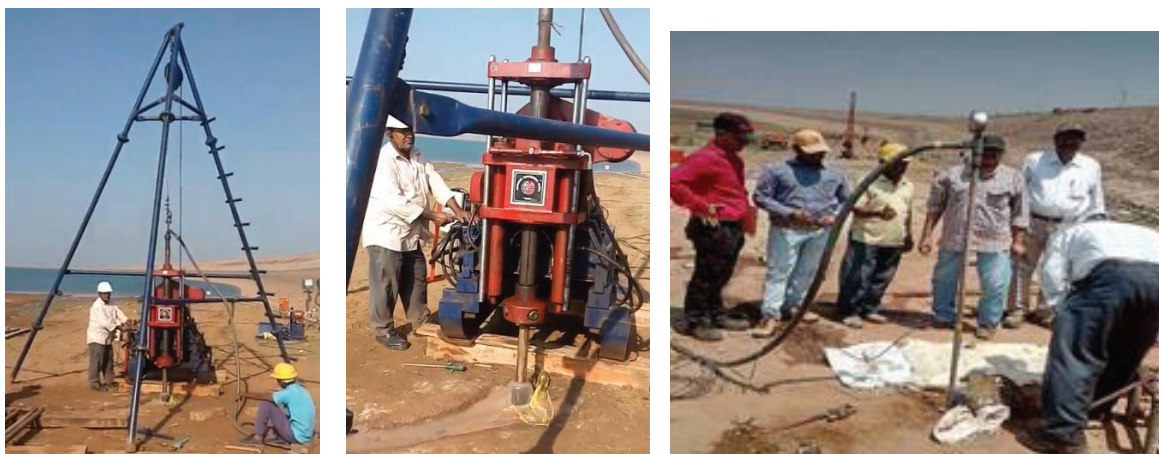
Photo 1 : 54 mm dia. Drilling work in progress, Photo 2 : In-situ permeability test in progress
