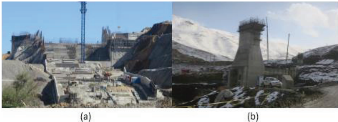
Figure 2 : (a) Spillway of KANISIB reservoir dam, April 2019. (b) Water intake tower of KANISIB reservoir dam, February 2019
