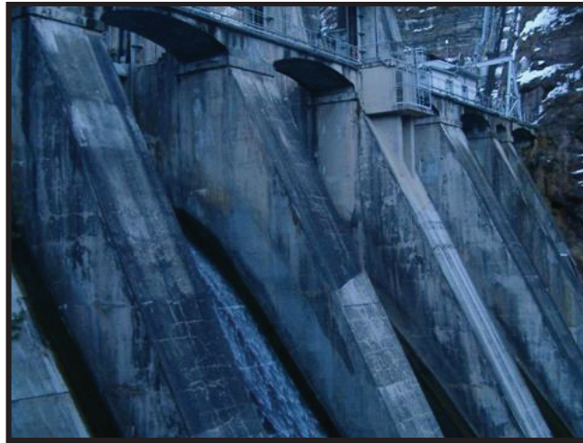
Figure 4 : Typical example of degradation caused by thaw/freeze cycles
