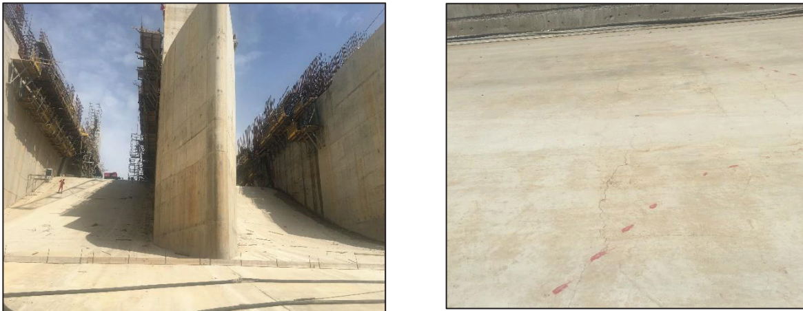
Figure 15 : Example of a cracked concrete of a spillway
