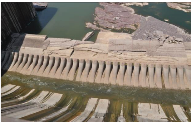
Figure 1 : Damages to bucket of main spillway
