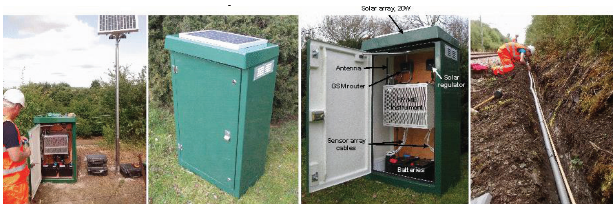
Figure 2 : PRIME system field deployments showing key components and sensors array installation.
