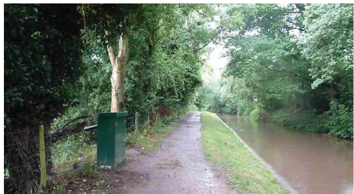
Figure 6 : PRIME system enclosure at the Llangynidr canal embankment monitoring site.
