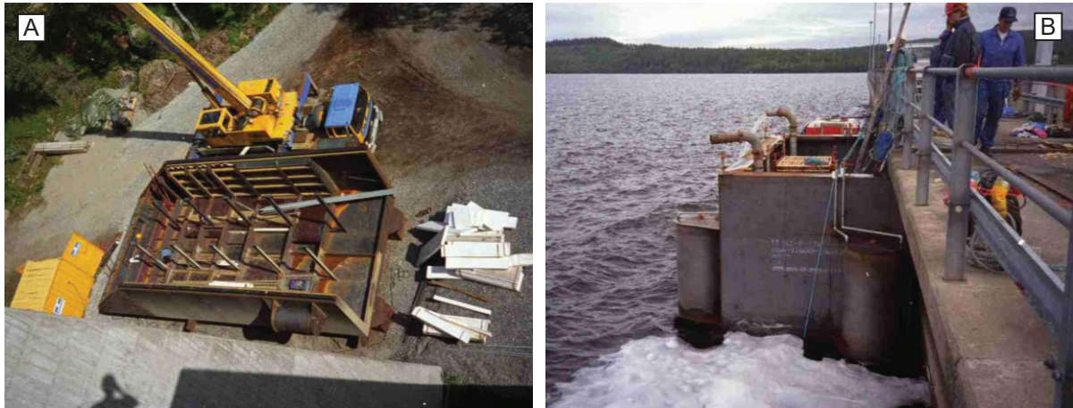
Figure 8 : The custom-made steel caisson used to allow work on the upstream face of the buttress dams (A). The caisson in place on the upstream side (B).
