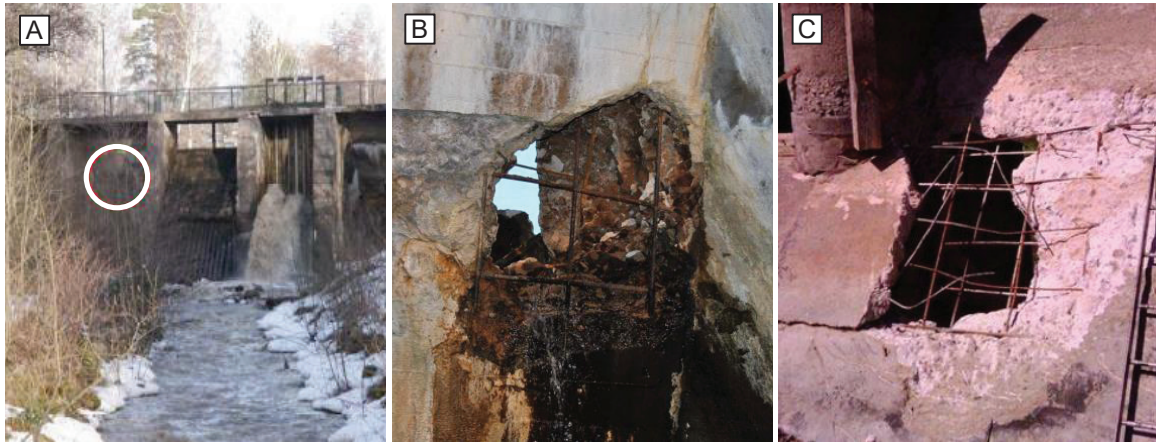
Figure 5 : A 70 year old buttress dam (A). In early spring, a hole appeared in the flat slab at a location where frost damage previously had been noticed on the downstream face (B-C).
