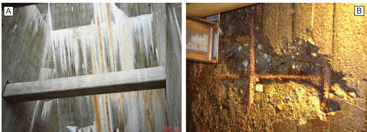
Figure 2 : Efflorescence on the downstream face due to leaching (A). Frost damage to the upstream face (B).
