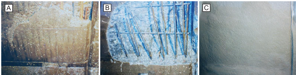
Figure 9 : Spalling of the concrete cover on the upstream face (A). Degraded concrete removed and reinforcement bars cleaned (B). Sprayed concrete applied (C).
