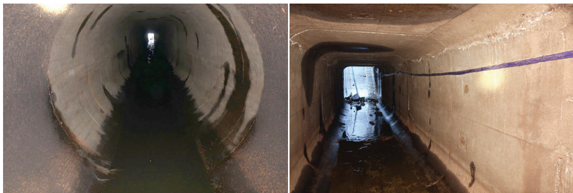
Figure 3 : Horizontal conduit – a short section of circular conduit (diameter 2.55 m) downstream of the bend (left); the major rectangular conduit (2.55 m in width, 2.55 m in height) with rounded corners running to the exit (right).
