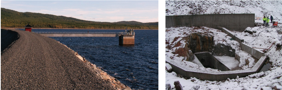
Figure 2 : Bottom outlet, with the intake tower in front of the embankment dam and the exit in the tailwater. The right photo shows the exit during a planned maintenance when the outlet was emptied of water.
