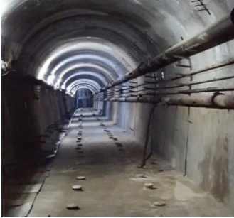
Figure 10 : Grouting Gallery with Legacy Infrastructure and Standpipes
