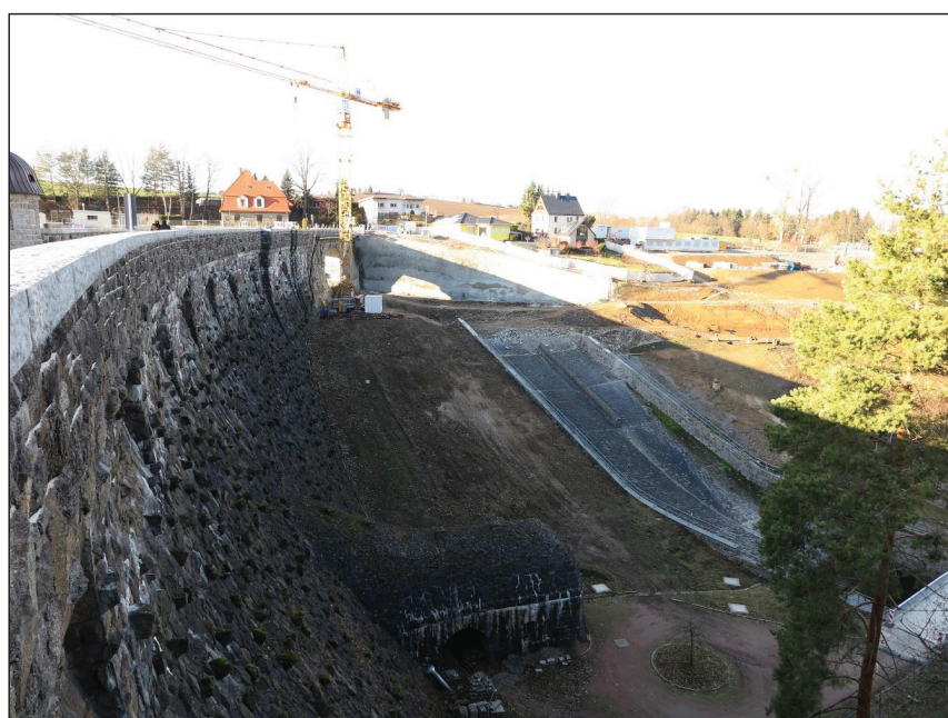
Figure 13 : Dam and Old spillway chute with location of diversion structure (to the right of the crane)
