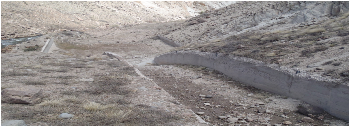
Figure 8 : Typical concrete freeze/thaw deterioration within the spillway discharge chute.
