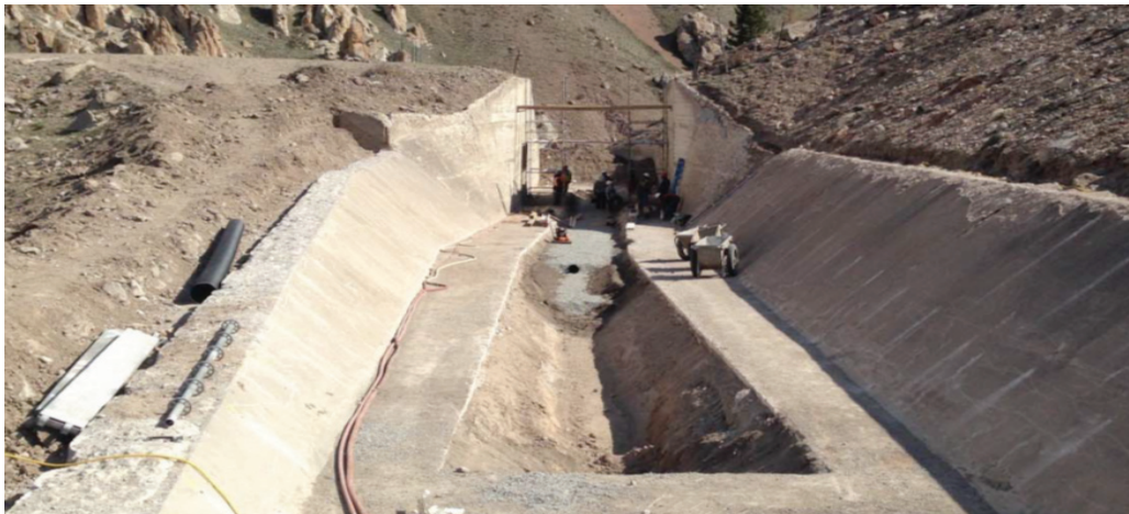
Figure 9 : Demolition of the spillway invert for installation of the underdrain system within the side channel spillway – side channel control section located to the left in the photo.
