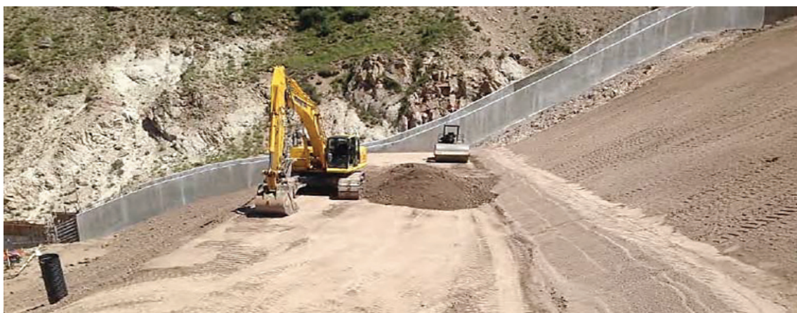
Figure 6 - Filter sand, gravel, and common fill placement for the filter system and stability berm.
