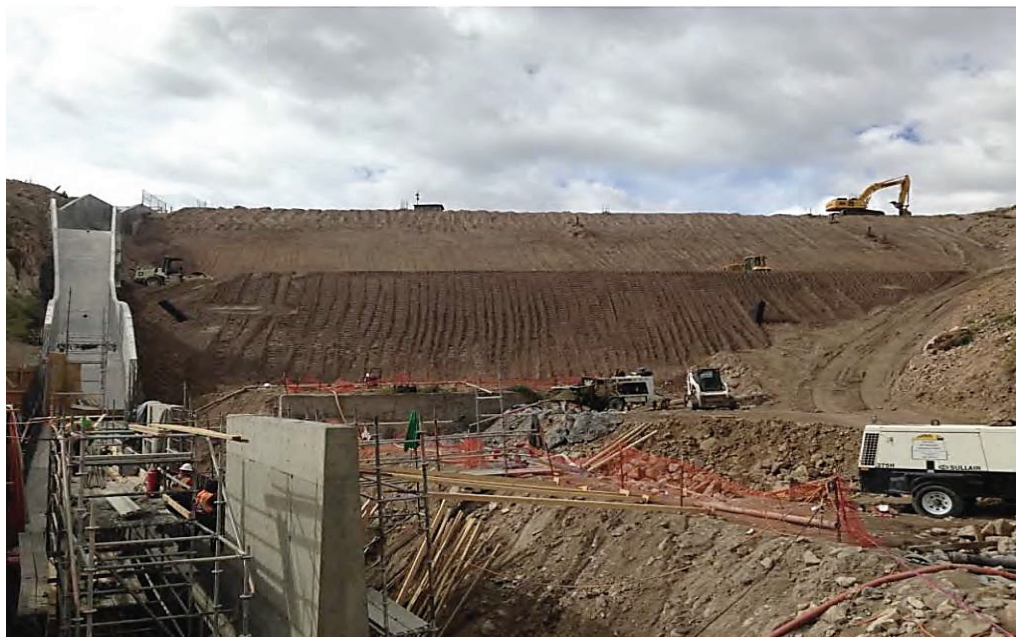
Figure 14 : Stilling basin to the left and the embankment stability berm under construction.
