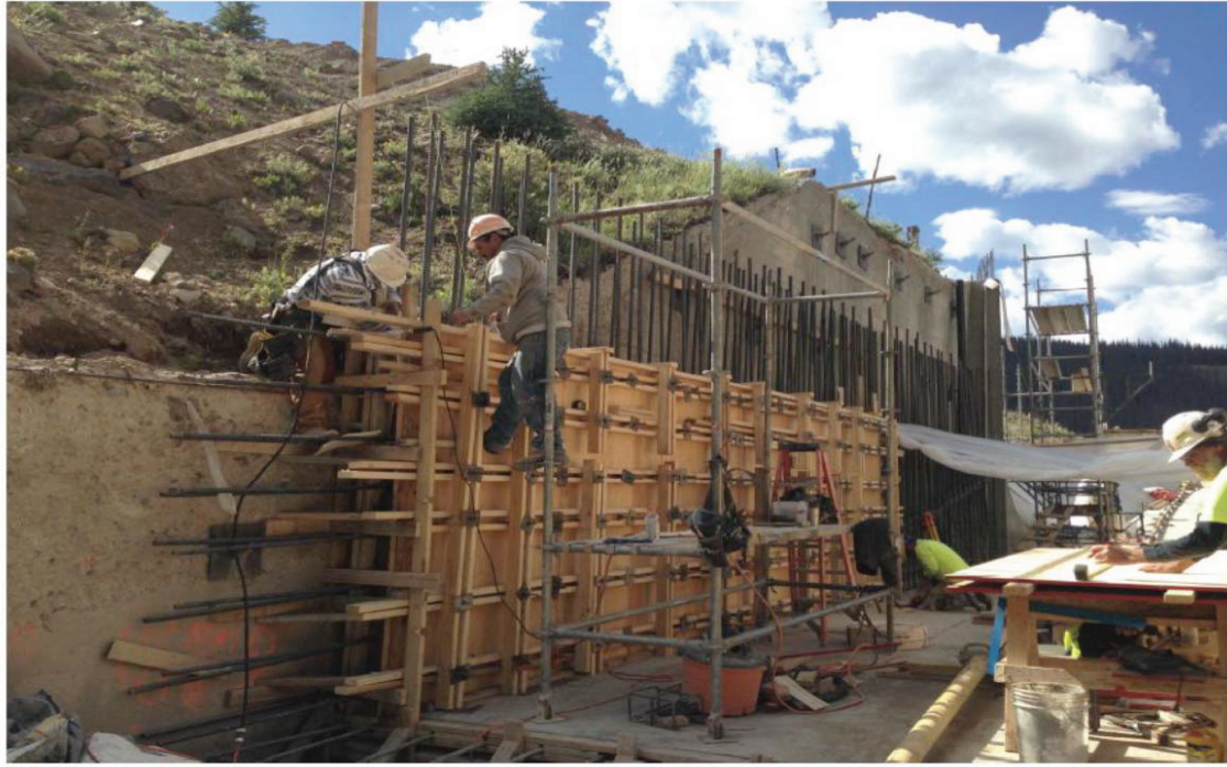
Figure 12 : Forming right chute wall using the existing wall as a form which helped reduce demolishing costs - the existing wall was characterized as soil for structural analysis.
