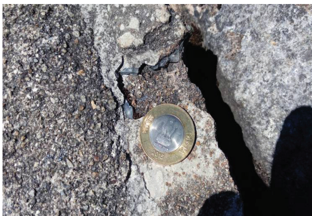
Fig. 3 : Broken tell-tale on the right abutment u/s
