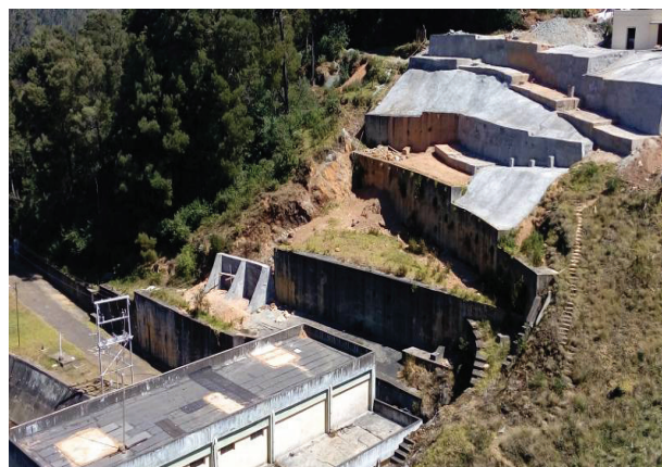
Fig. 4 : Slope protection/retaining wall with weep holes on the d/s right abutment above PH
