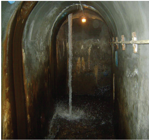
Fig. 1 : Ingress of water into drainage gallery by piping
