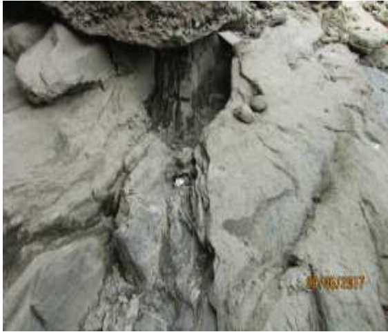
Fig. 5 : Eroded foundation of Pier- 3, view from u/s to d/s facing towards left bank
