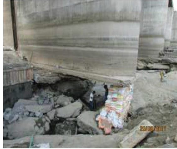
Fig. 6 : Shear plane day lighted at foundation of pier-3 the sheared/weathered rock scooped out by water action
