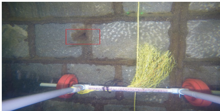
Figure 3 : Anomaly found using EyeROV TUNA during a Dam Inspection
