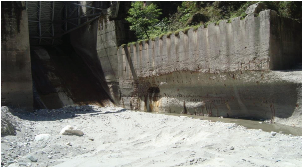
Photograph 6 : (Damaged Left Training wall)
