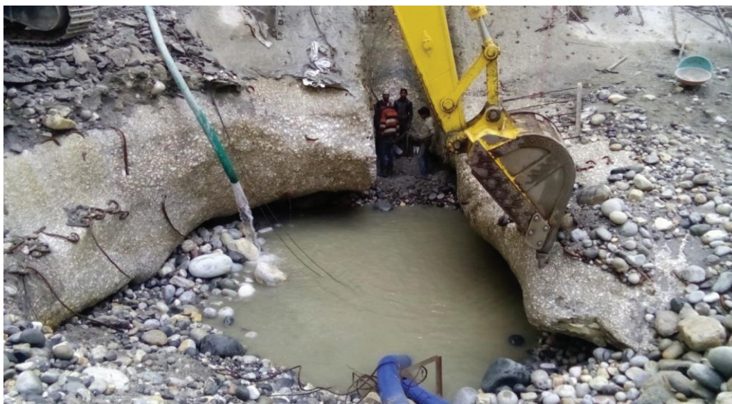
Photograph 7 : (Cavity in Slotted Roller Bucket)
