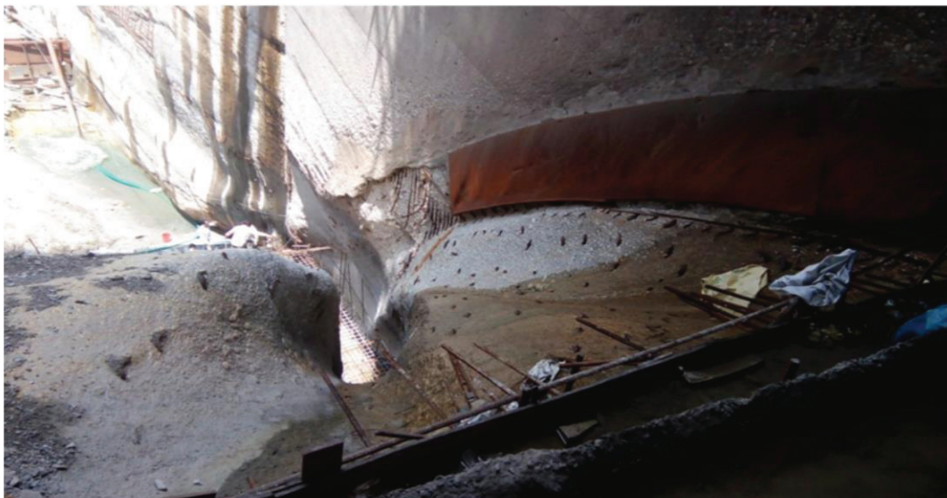
Photograph 2 : Shows the damages in Spillway bay no-1
