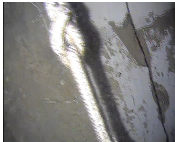
(a) Before repair
