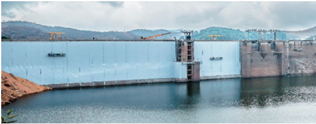
Figure 8 : Overview of the dam with nearly 20% of the upstream face installed with Geomembrane system & Optical Fiber Cable.
