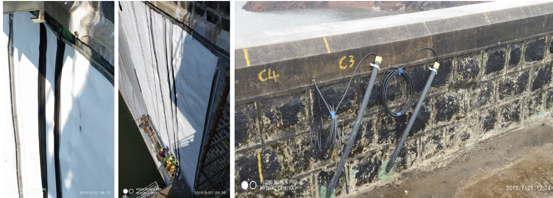
Figure 10 : From Left to right, Fiber Optic cable positioned above the geotextile, geogrid protecting the fiber cable and an external protective pipe covering the exposed optical fiber cable at the crest
