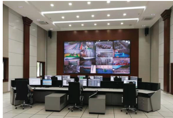
Figure 6 Centralized Control Center
