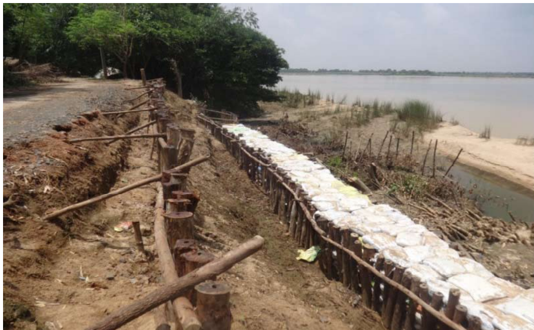
Figure 5 : Restoration of subsidence of right bank of river Damodar at Nabagram, Burdwan as obtained from Flood Report 2015 flood, I & W Dept. West Bengal
