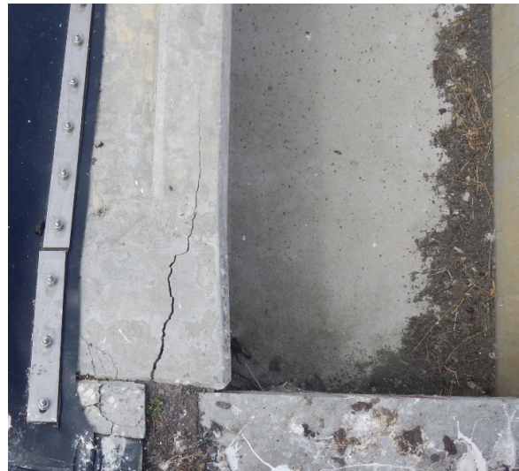
Figure 20 : Damage of concrete at outlet
