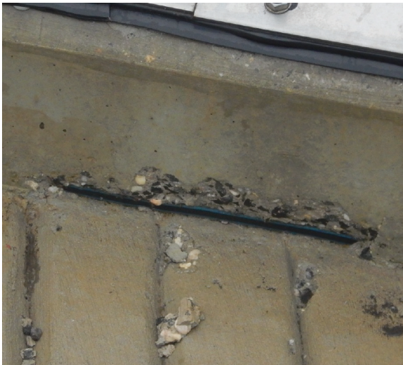
Figure 19 : Damage of concrete at boat ramp
