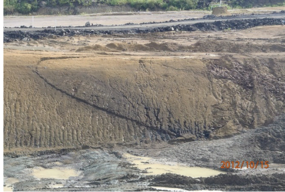
Figure 5 : Example failure of outboard core trench slope
