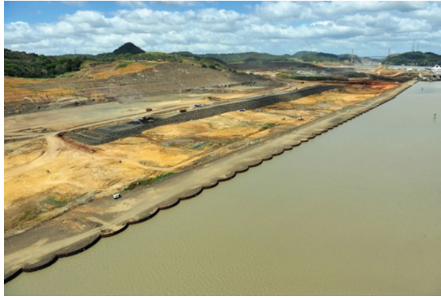
Figure 4 : Dam 1E foundation with cellular cofferdam in foreground, PAC excavation in background, and rockfill shell on the inboard dam foundation
