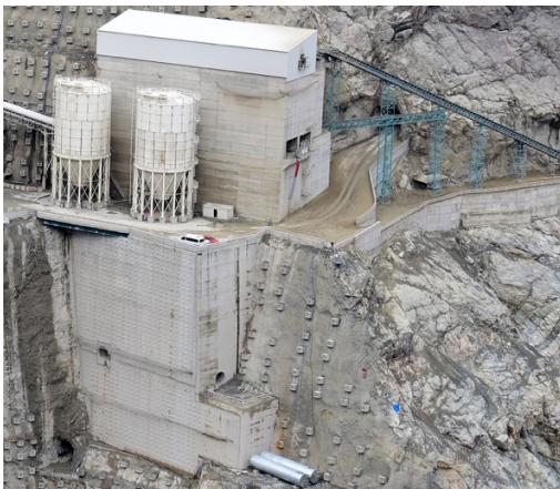
Figure 5. The first concrete block supporting temporary works at the top of the left abutment
