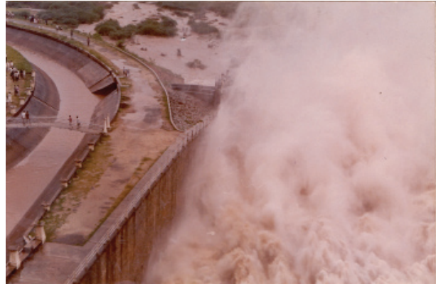
Figure 8 : Dantiwada Dam – endangered due to heavy flood
