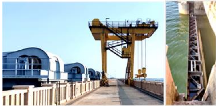
Figure 8. Narayanpur dam new gantry crane and set of stop logs.
