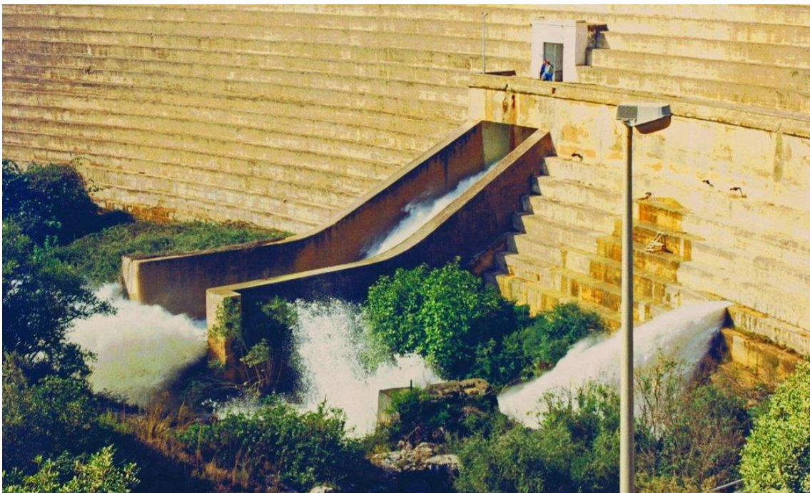
Figure 2. Uncontrolled outflow next to the bottom outlet detected during overtopping.
