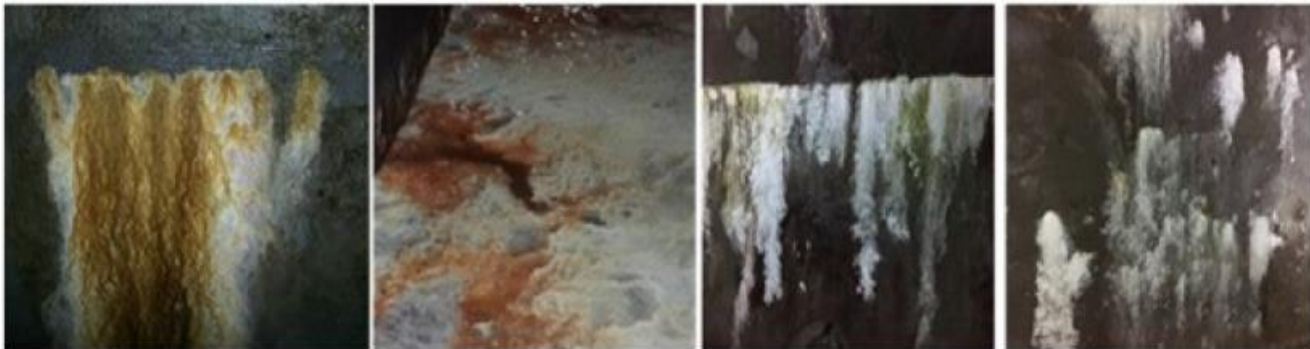
Fig. 8 : Leaching of Lime
