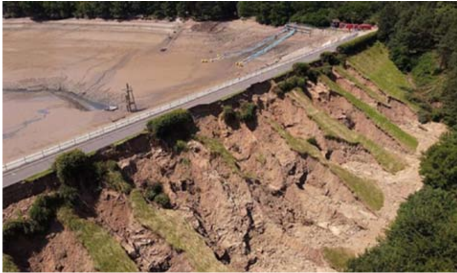
Fig. 2 : Overtopping of Steinbach dam in Germany (14.7.2021). The paved road across the crest saved the dam.
